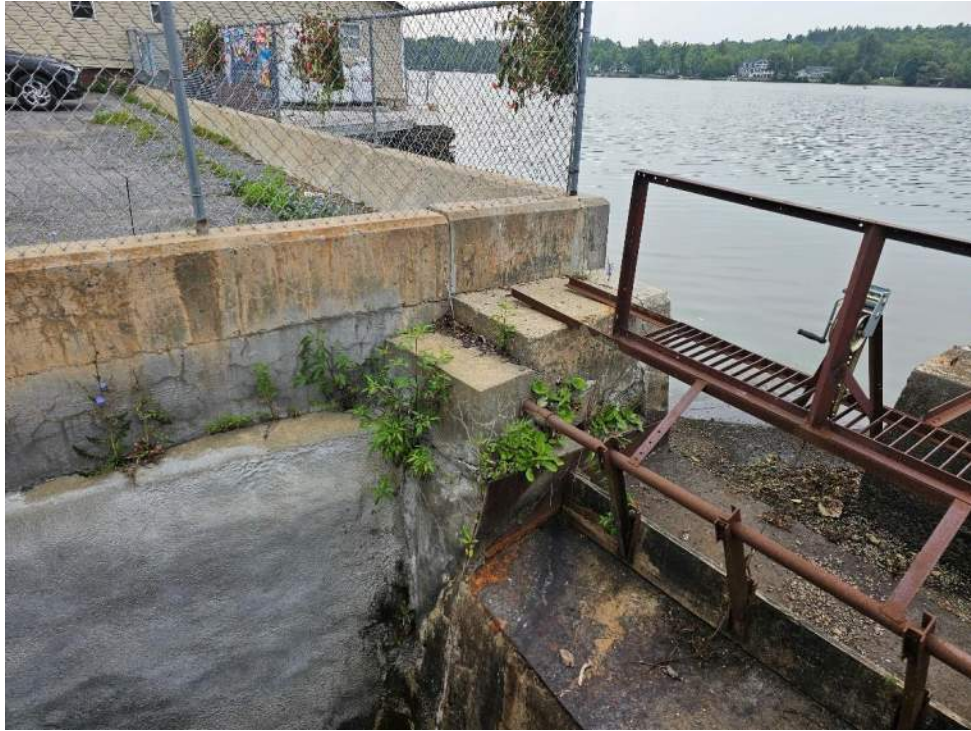
Spillway/Flashboards – In Lowered Position
