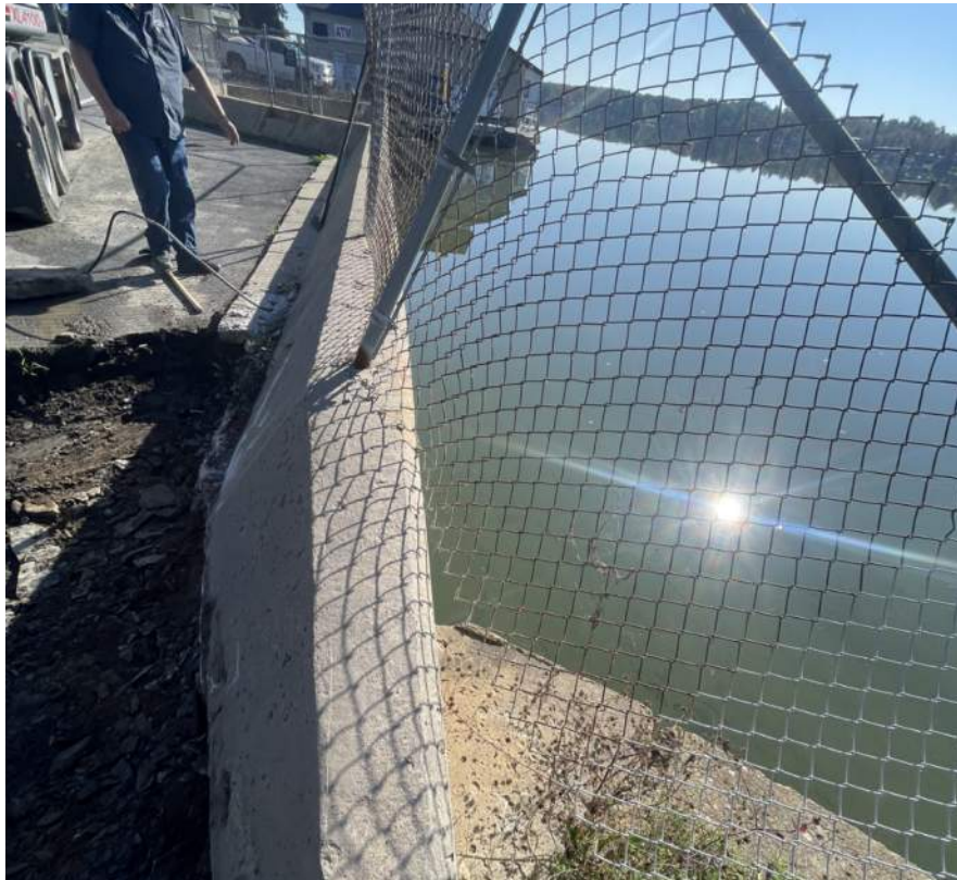
Lake water surface elevation below sinkhole area
