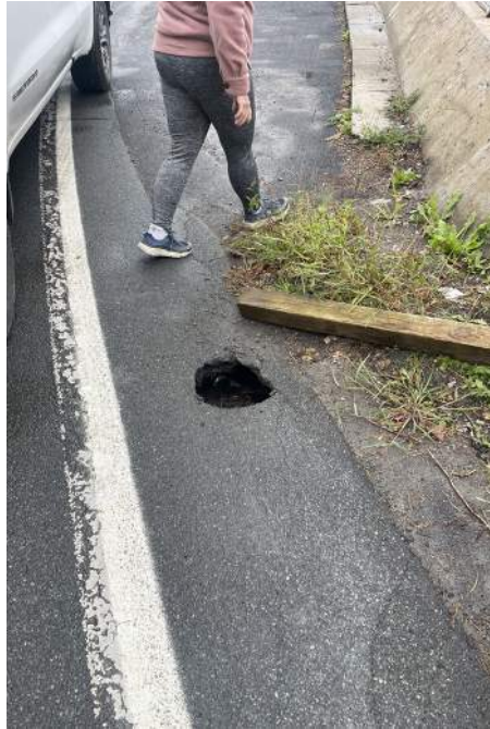
Sinkhole behind western dam abutment as discovered on 9/30/23
