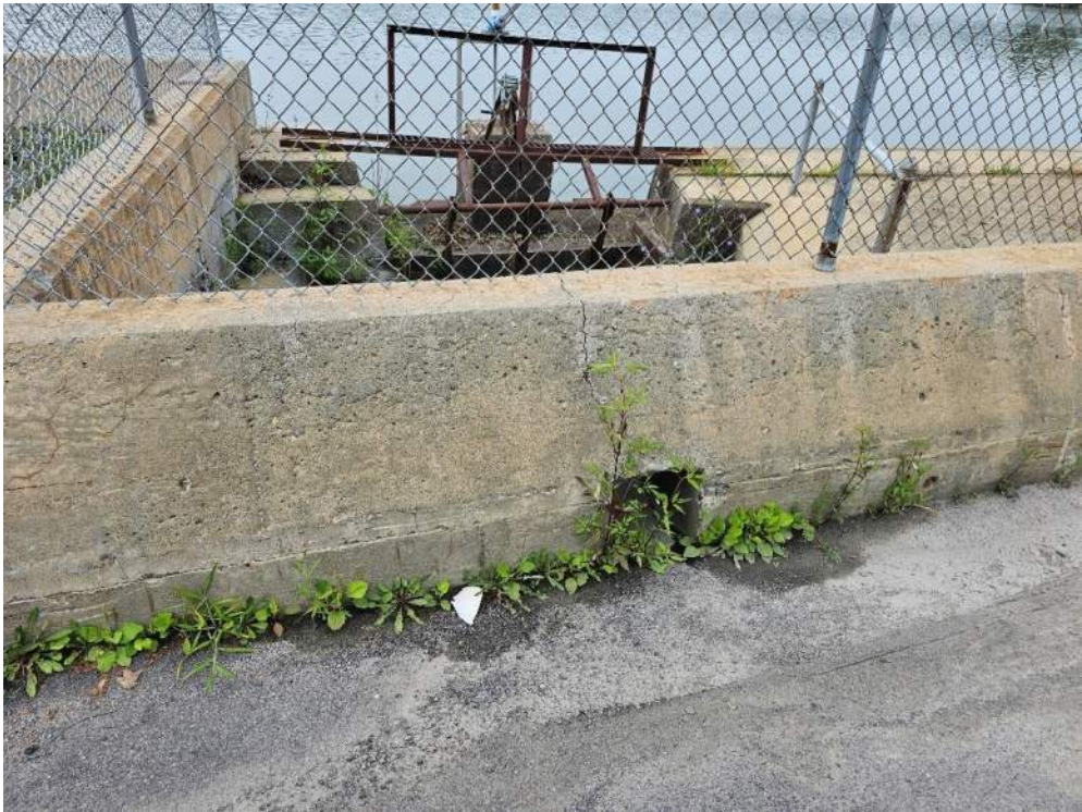
Downstream Face of Drop Inlet – Crack Above Drainage Slot
