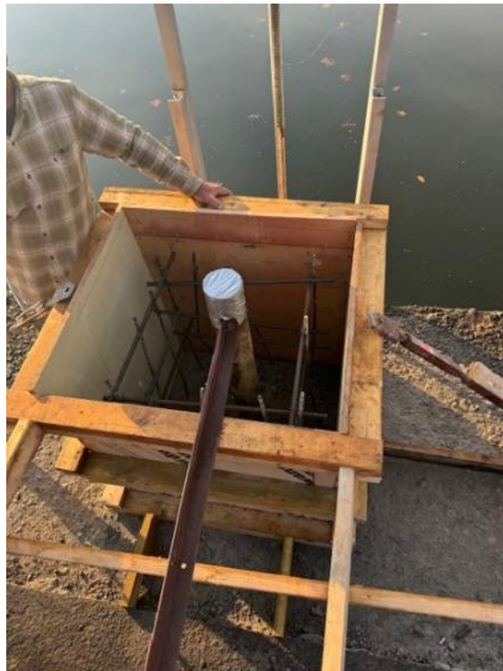
Forms and new rebar for new concrete around abandoned low level outlet valve
