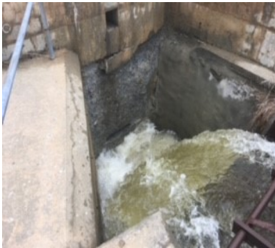
Deteriorated Spaulding Spillway
