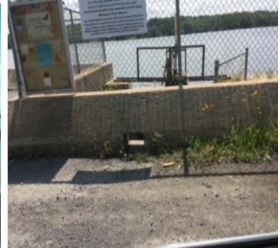
Road in front of Dam Holding Water causing deterioration to dam face
